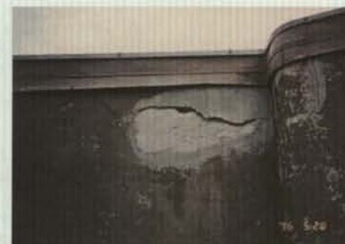
Fig. A14 above Deep cracking and peeling paint on roof penthouse stucco
