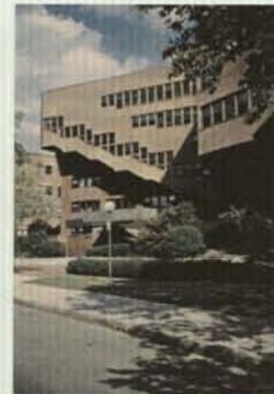
Fig. A11 North elevation exhibiting dark areas of stucco under window corners where white surface aggregate is eroded
