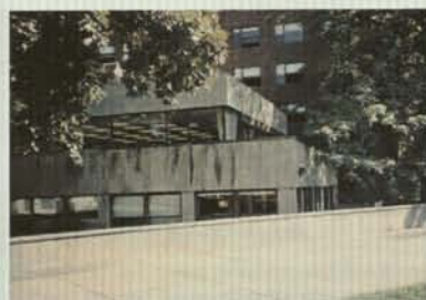
Fig. A17 top right Biological growth staining on limestone sheathing, south and west elevations of dining hall
