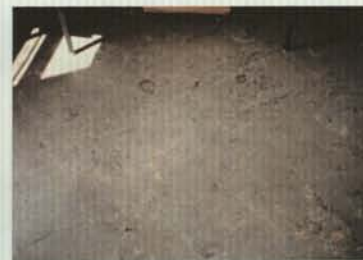
Fig. A28 Asphalt tile deterioration
