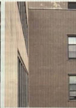
Fig. A13 Cracking and staining of the north elevation stucco
