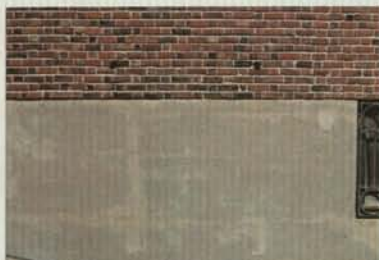
Fig. A5 Discoloration of concrete along joints of the formwork
