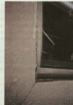
Fig. A12 Finish coat of stucco completely abraded exposing brown coat underneath
