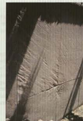
Fig. A15 right Surface erosion on the limestone sheathing, west elevation of dining hall
