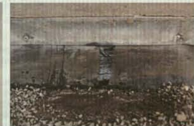
Fig. 117 Water behind base flashing Level "F"
