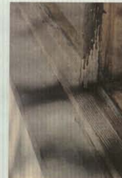
Fig. 129 Detail of wood windows showing checked sills and deteriorated finish.
