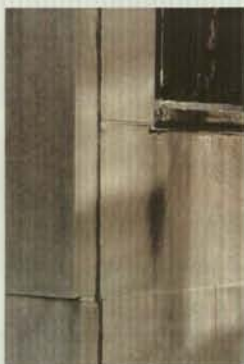
Fig. 83 Limestone detail showing failed sealants and fungal growth
