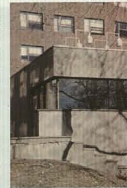
Fig. 68 Moon Garden Pavilion with spalling concrete terrace and eroded soil.
