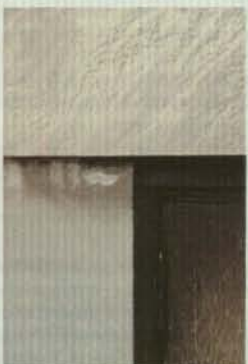
Fig. 84 Limestone detail showing soiling and sugared stone
