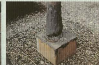
Fig. 119 Failed pitch pocket Level "F"
