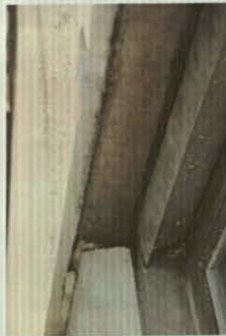
Fig. 89 Exposed lintel behind limestone at Pavilion
