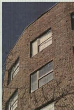
Fig. 124 Typical south facade windows (and damaged roof coping)
